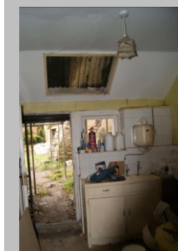
In the 50s Mr Tett put the hot water heater in and Mrs Tett did ironing by plugging in to the light socket.
